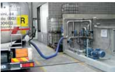
RECOVERY OILS PLANT
